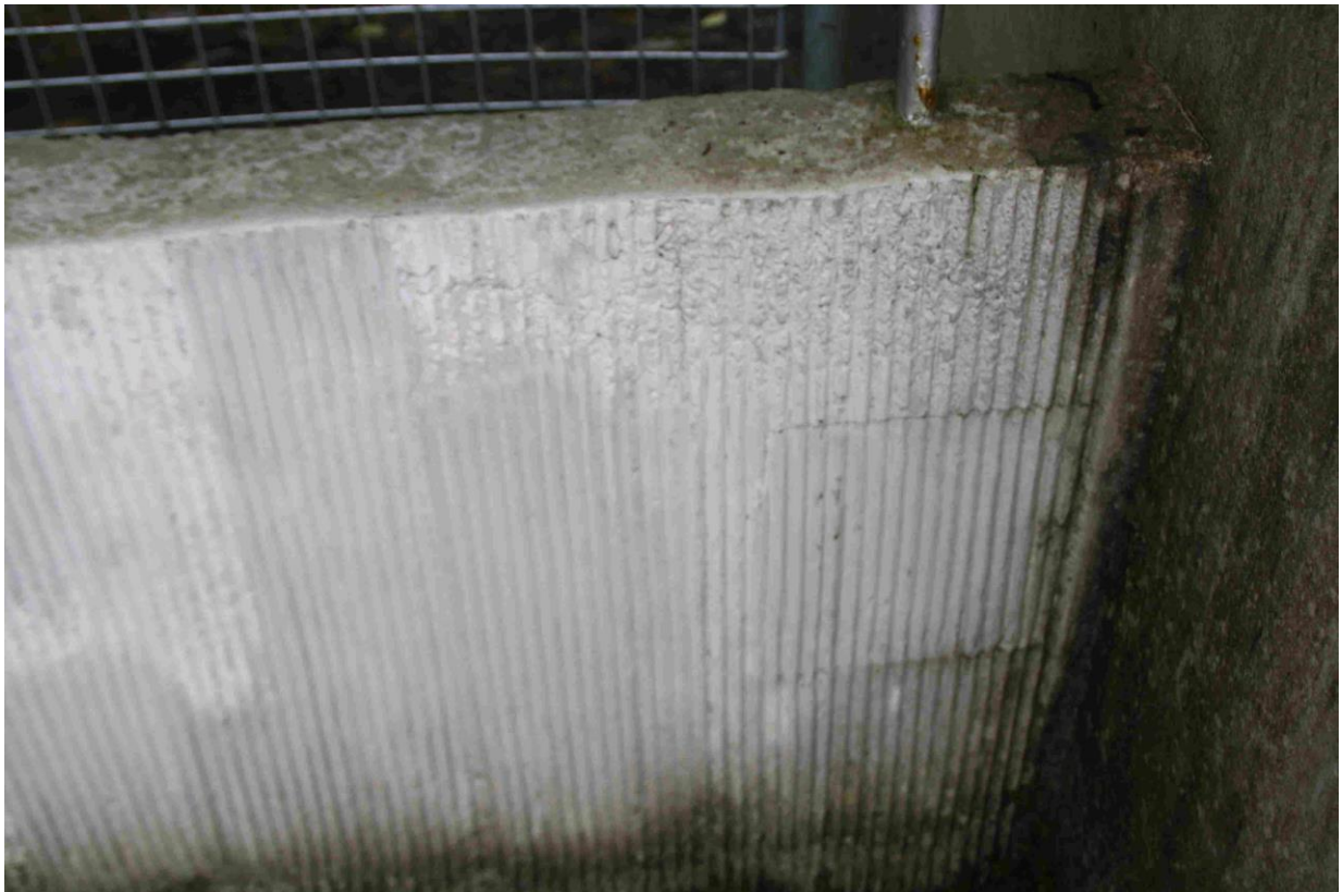
Figure 6 Classic shrinkage cracks noted around a square repair to the fluted section of the 1 st floor wall.
