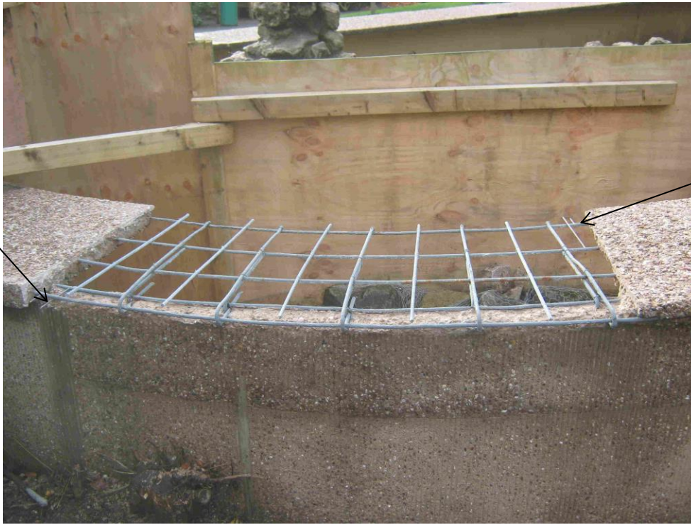
Figure 13 Broken out section at the back of the Meerkat Enclosure (2015 - prior to repairs) showing the four stainless steel test points (right front and left back) attached to the different rebars.
