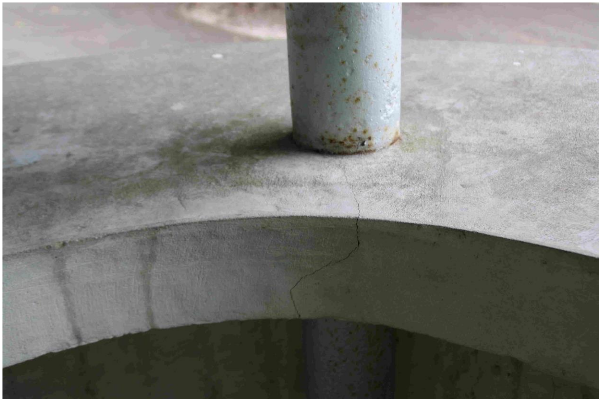
Figure 2 Fine crack leading out from the steel column, possibly due to differences in thermal expansion between the steel and the concrete.
