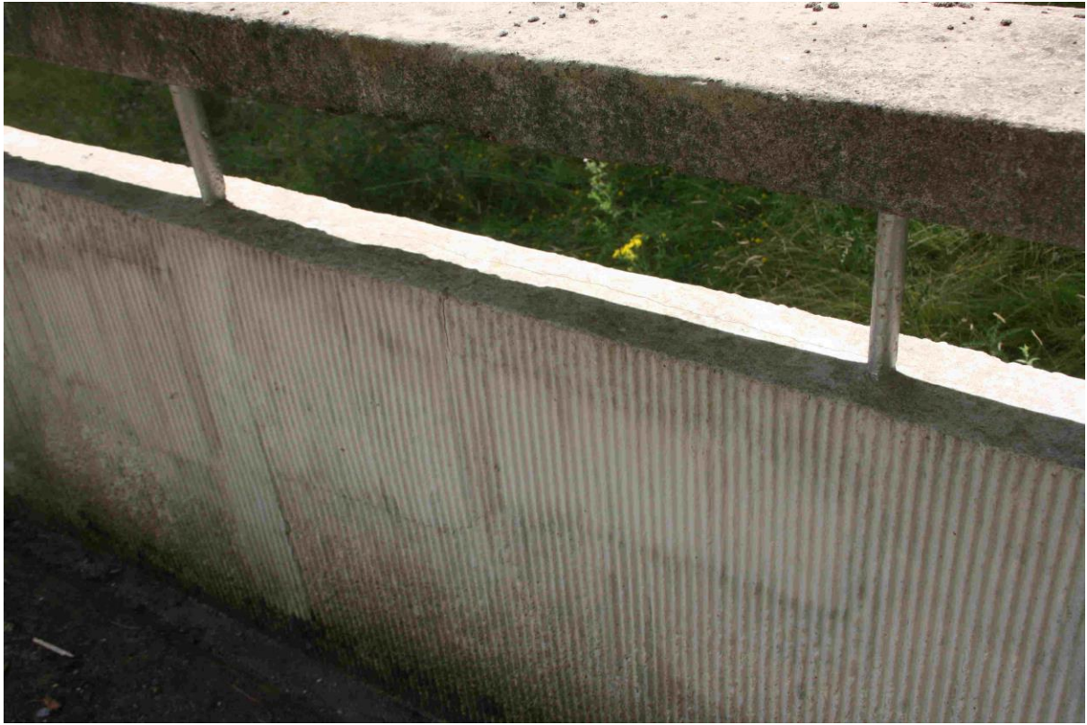
Figure 5 Another crack noted to a repaired parapet wall to the Bear Ravine.
