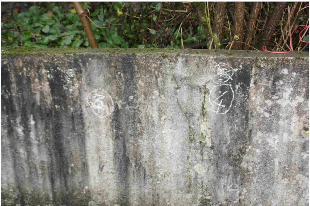
Figure 8 View of the small patch repairs (3 and 4) on the inner wall at 1 st floor level. Patch 3 was made using a proprietary repair mortar and patch 4 was made using a like-for-like concrete repair. Note – shrinkage and moss growth (in cracks) for patch 4.
