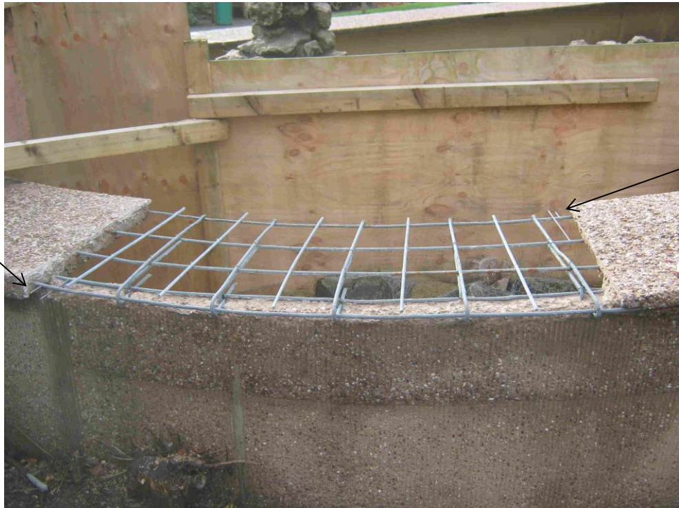
Figure 13 Broken out section at the back of the Meerkat Enclosure (2015 - prior to repairs) showing the four stainless steel test points (right front and left back) attached to the different rebars.
