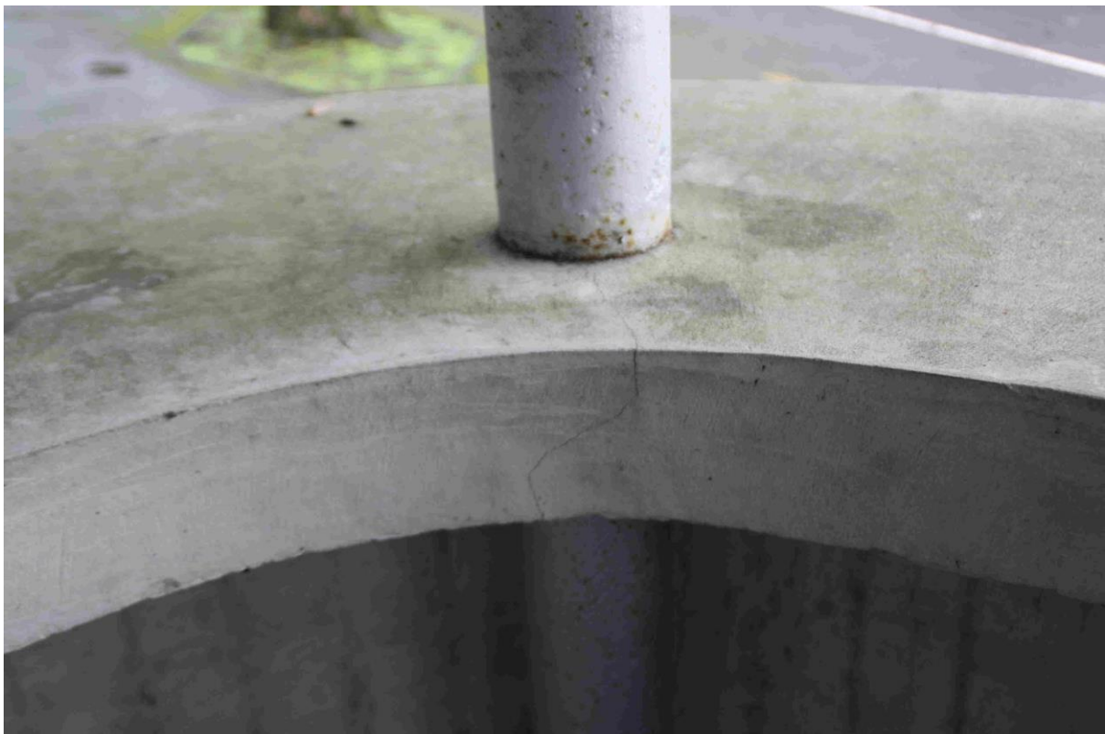
Figure 2 Fine crack leading out from the steel column, most probably due to shrinkage of the repair concrete.
