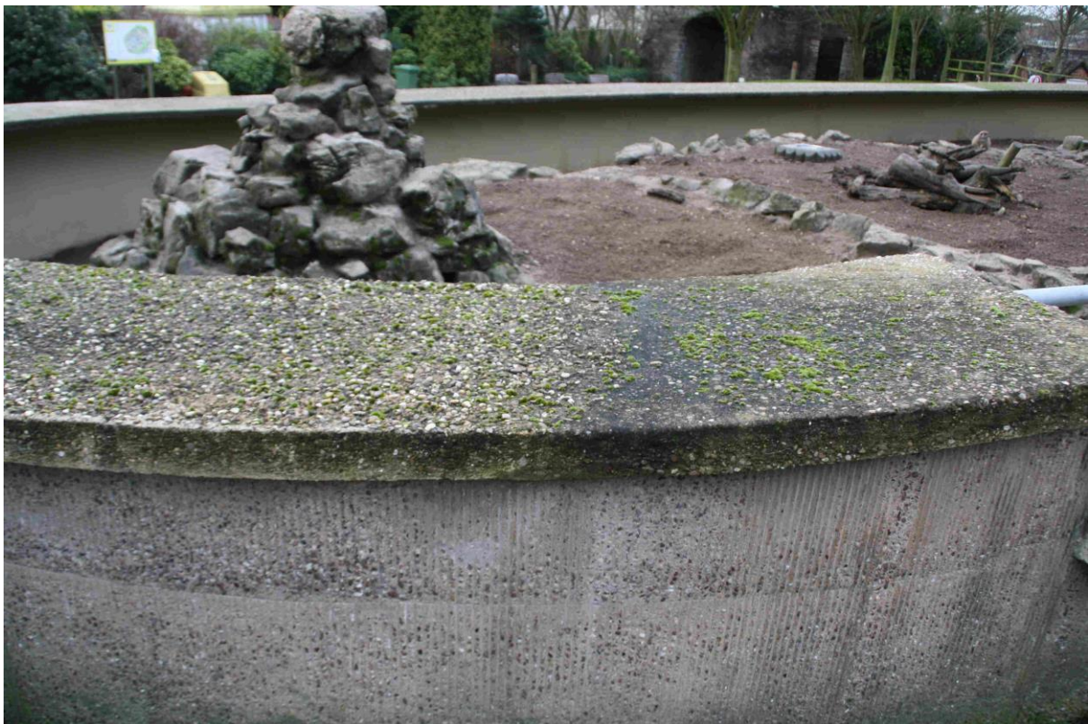
Figure 14 View of the repaired top of the wall showing it almost fully blending in after 5 years exposure.
