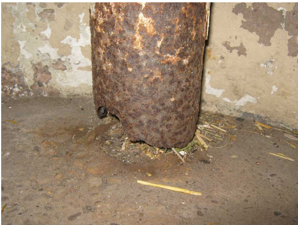
Figure 7: Corrosion damage to the base of a steel pillar within the Kiosk.
