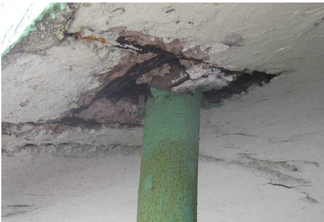
Figure 8: Corrosion damage to the underside of the sinusoidal roof of the entrance.
