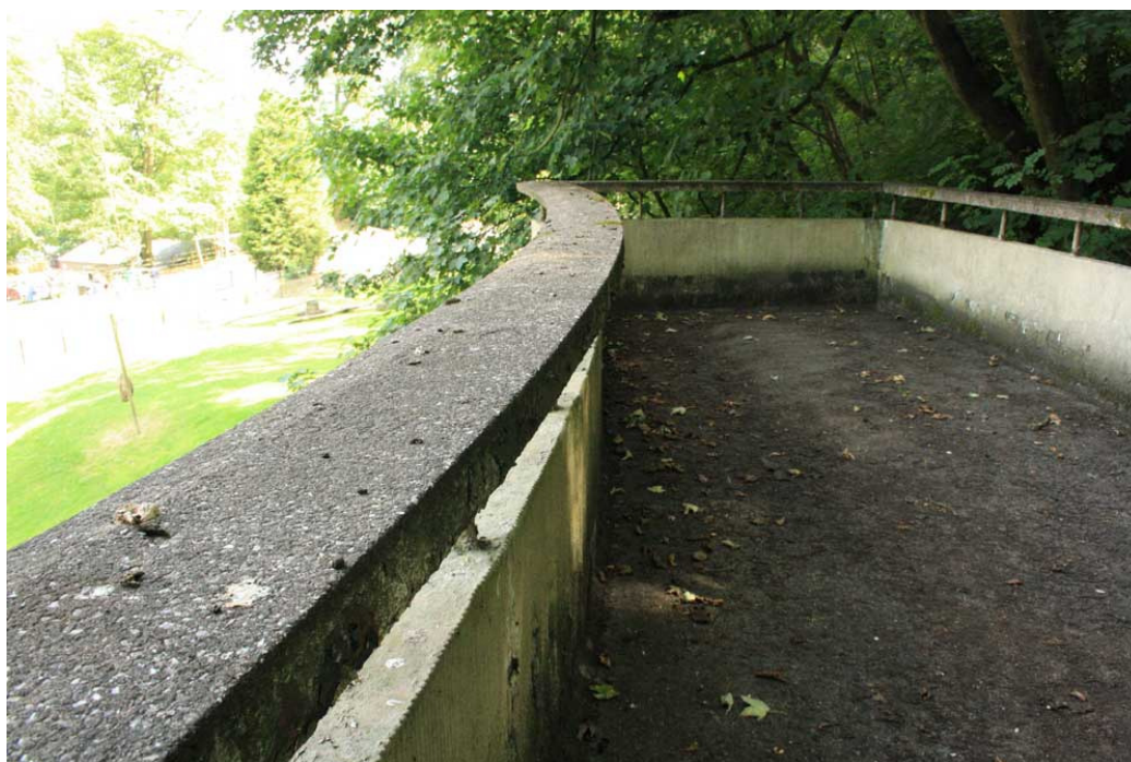
Figure 2: Weathering of the cementitious components of the concrete has left the aggregates exposed on the Bear Ravine's balustrade rail.
