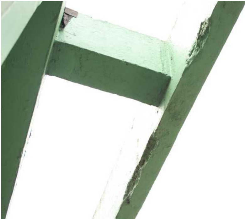
Figure 9: Localised damage to the flying edge beam of the Safari Shop.
