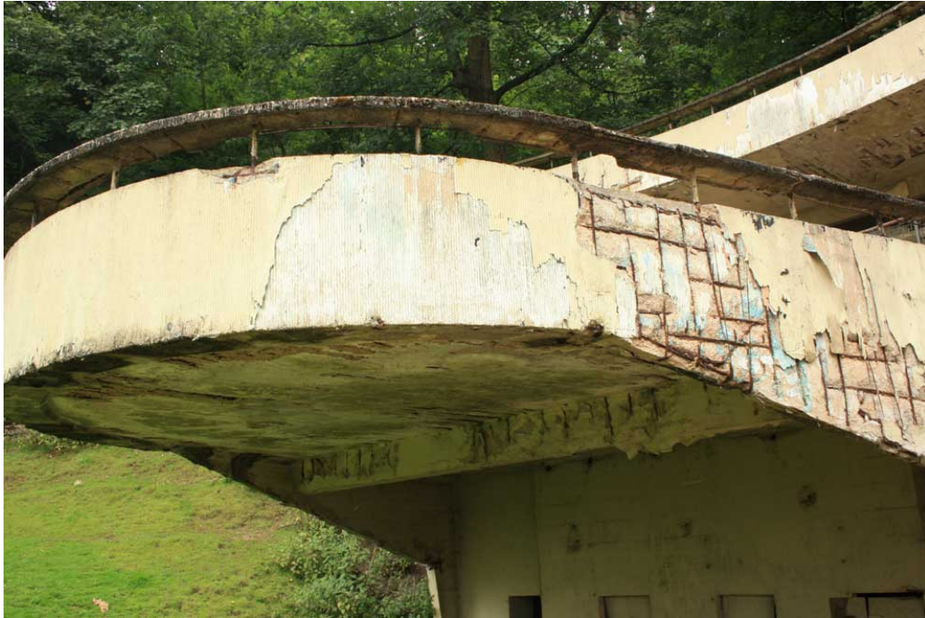
Figure 5: The cantilevered balcony of the Bear Ravine was in a particularly poor condition.
