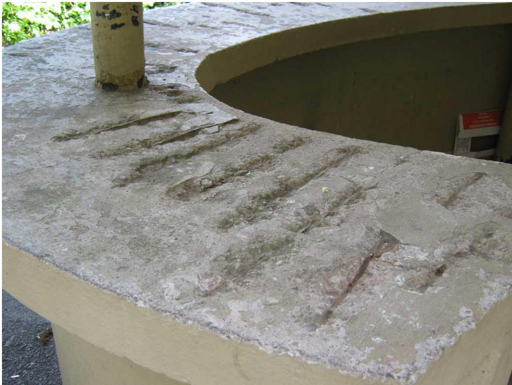
Figure 6: Corroding reinforcements are exposed due to low concrete cover on the Kiosk worktop.
