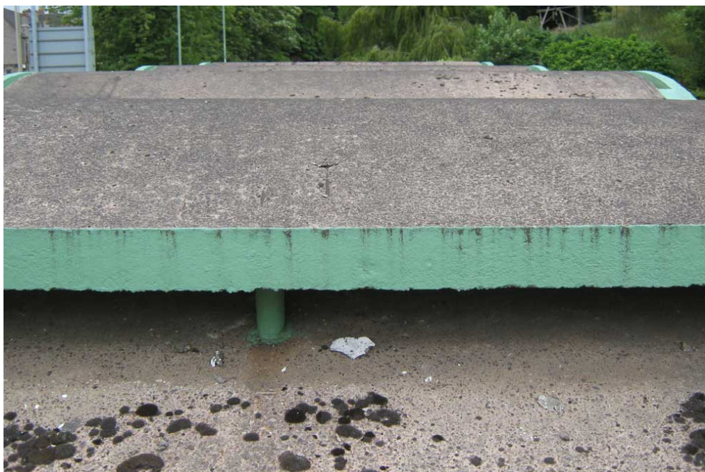
Figure 1: The weathering of the uncoated curved roofs of the entrance structure as compared with the unweathered surface of the underlying adjacent roof curve.
