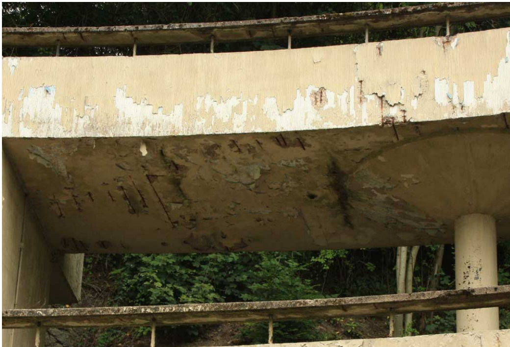
Figure 4: The soffit of the upper platform showed significant corrosion of the low-lying reinforcements.
