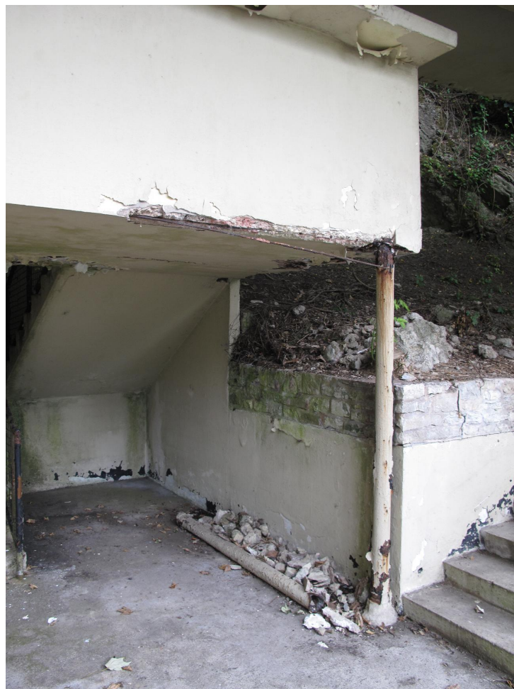
Failure of steel posts supporting stair landing (before temporary support was installed)
