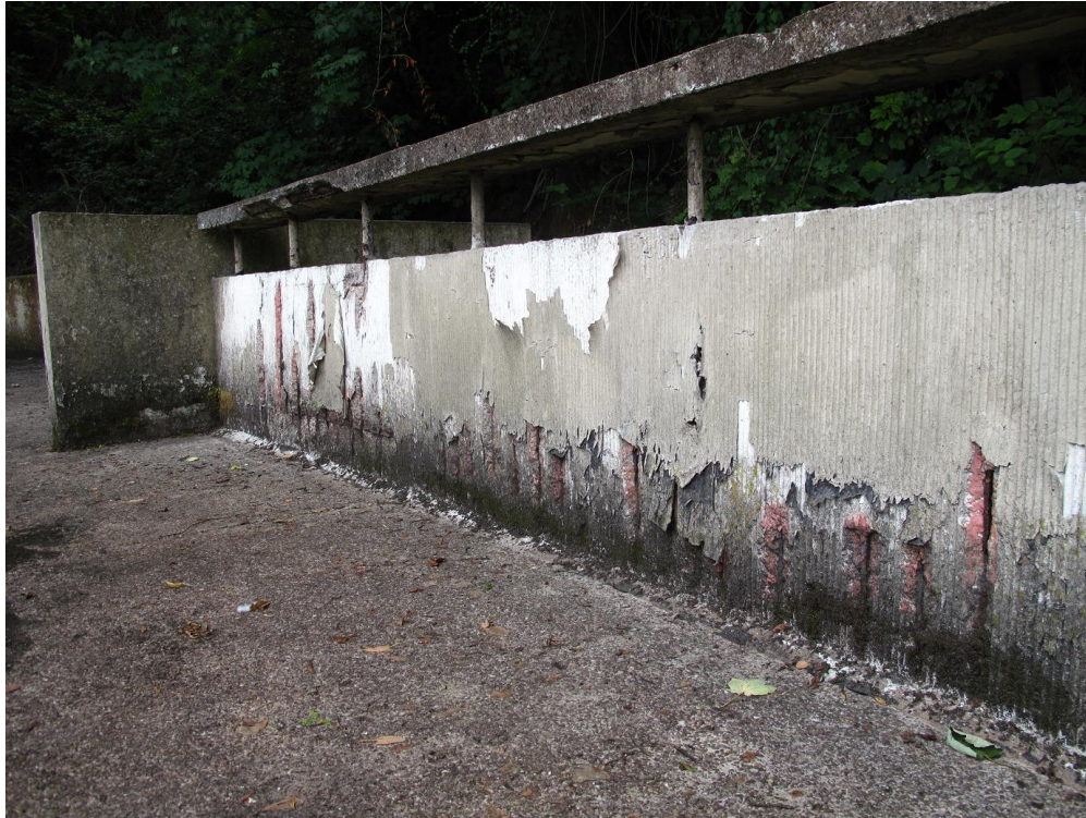
Corrosion to parapet wall to high level walkway
