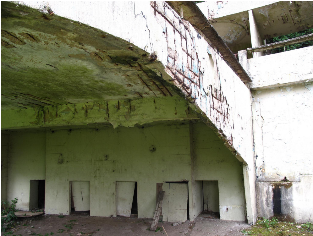
Extensive corrosion to parapet wall which supports and anchors the cantilevered viewing platform
