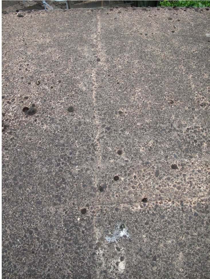
Longitudinal crack in top of roof slab
