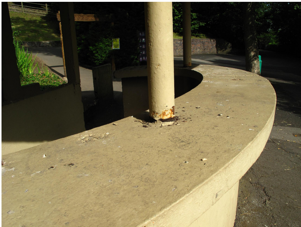
Corrosion to steel post at reinforcement in counter
