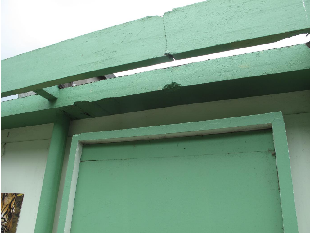
Spalled concrete edge beam at roof level
