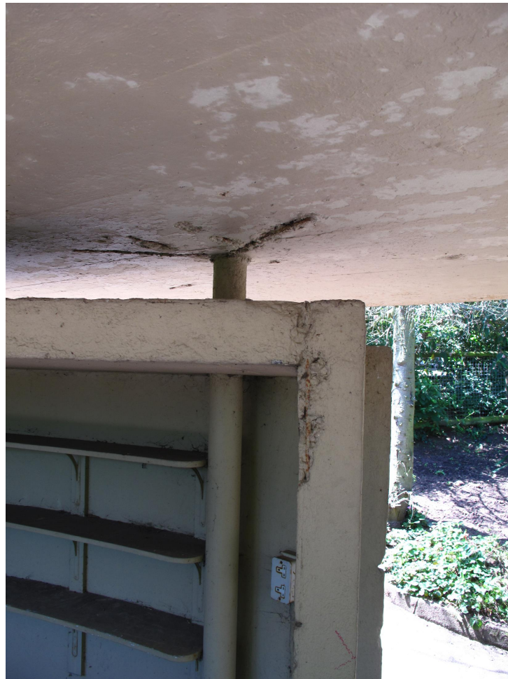
Corrosion to bars in roof slab around top of posts
