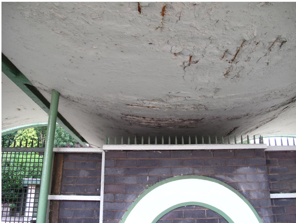
Corroded reinforcement and spalled concrete to underside of roof slab
