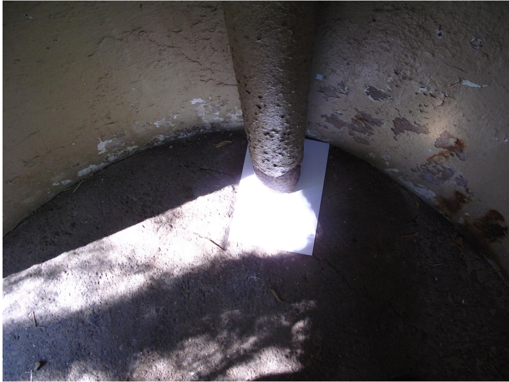
Base of steel post has completely corroded
